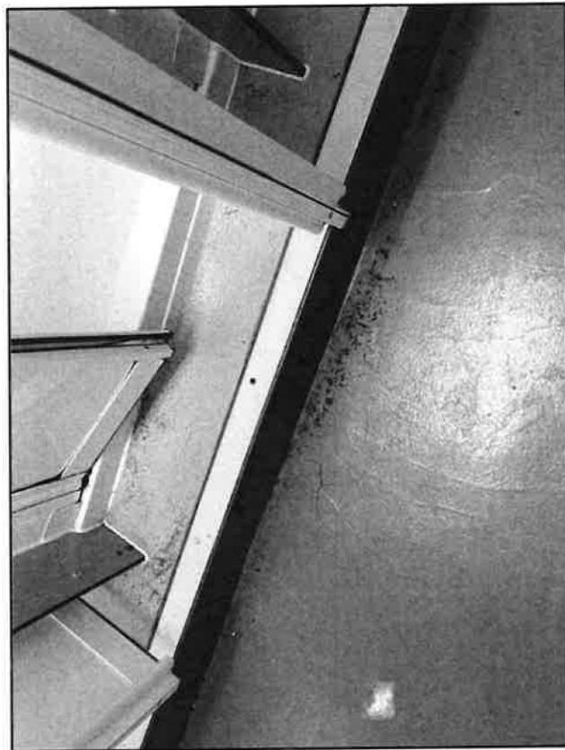
066. Mould to flooring within female changing area/shower block
