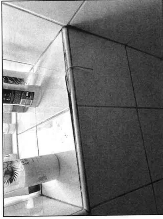
070. Defective silicone between tiles within G27 equipment store
