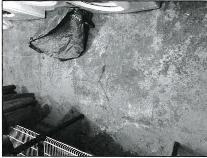
075. Cracking to concrete floor within 029 Laundry
