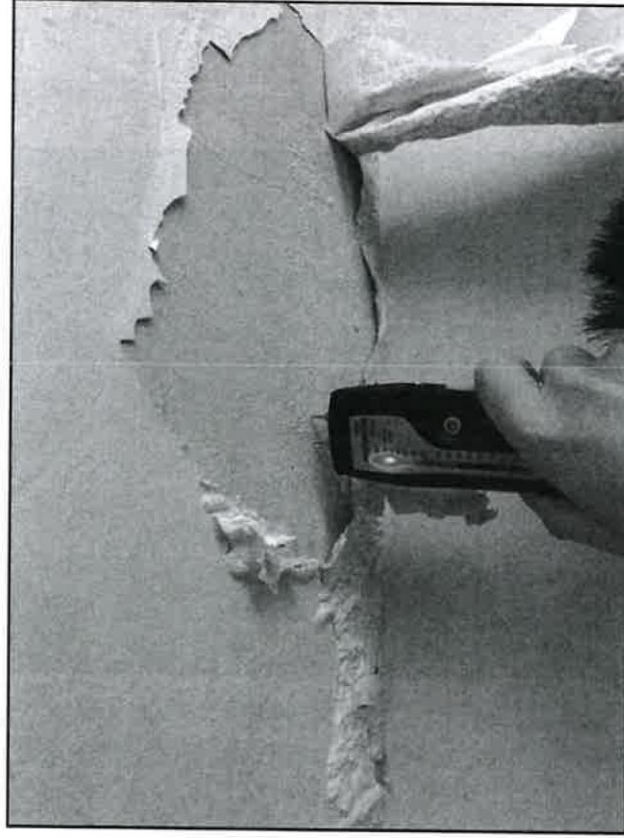
059. High damp meter readings to ceiling at underside of stairs adjacent to G14
