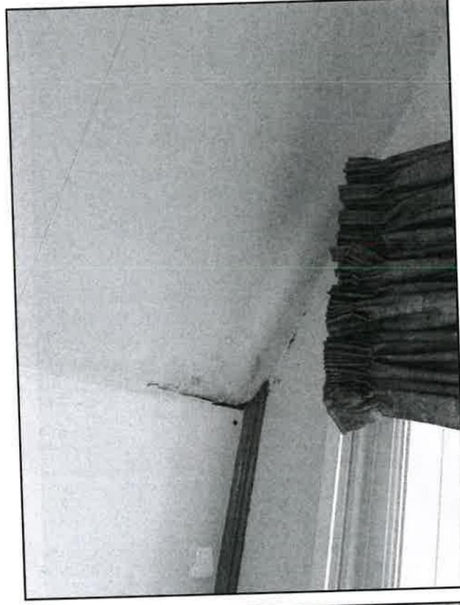
080. Mould to ceiling above bunk bed within Grasmere bedroom
