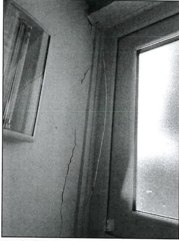
060. Crack to ceiling adjacent to external door at underside of stairs adjacent to G14
