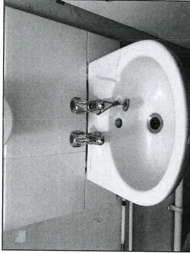
064. Mould affected and defective silicone behind sink of female changing area
