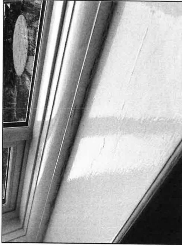
055. Defective seal to sill within Lounge
