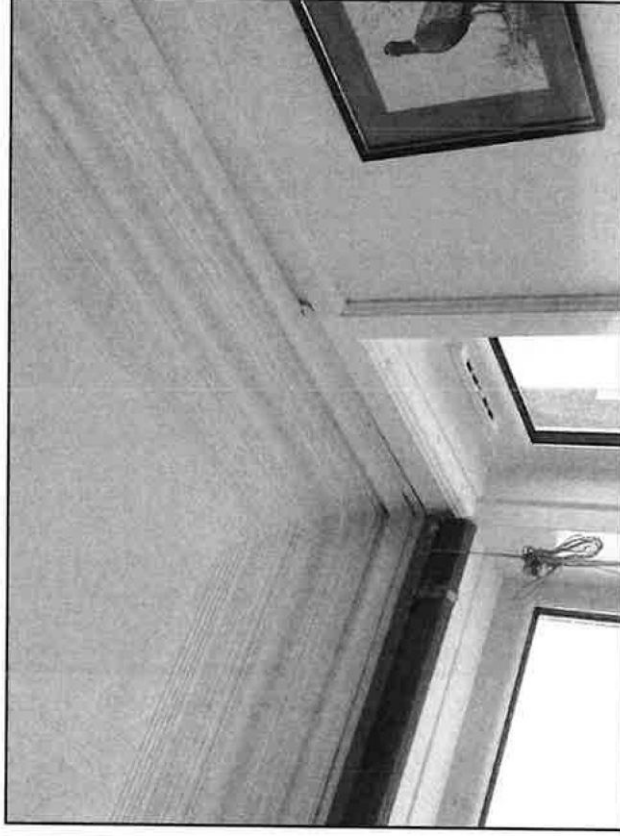
056. Horizontal non-structural crack above window of
