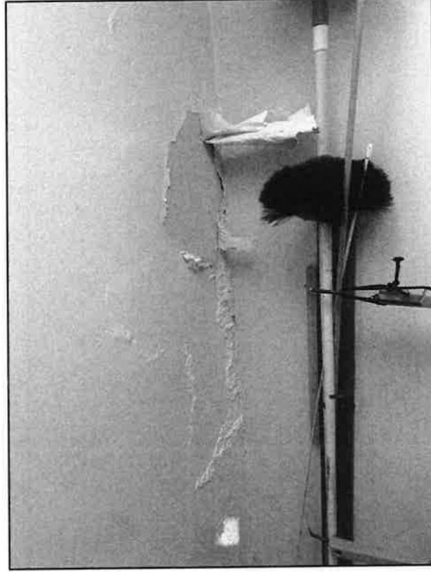
058. High damp meter readings to ceiling at underside of stairs adjacent to G14
