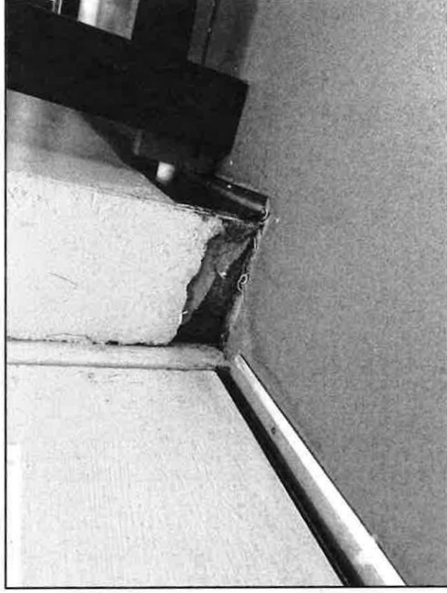
074. Example of missing section of PVC flexible skirting within conservatory
