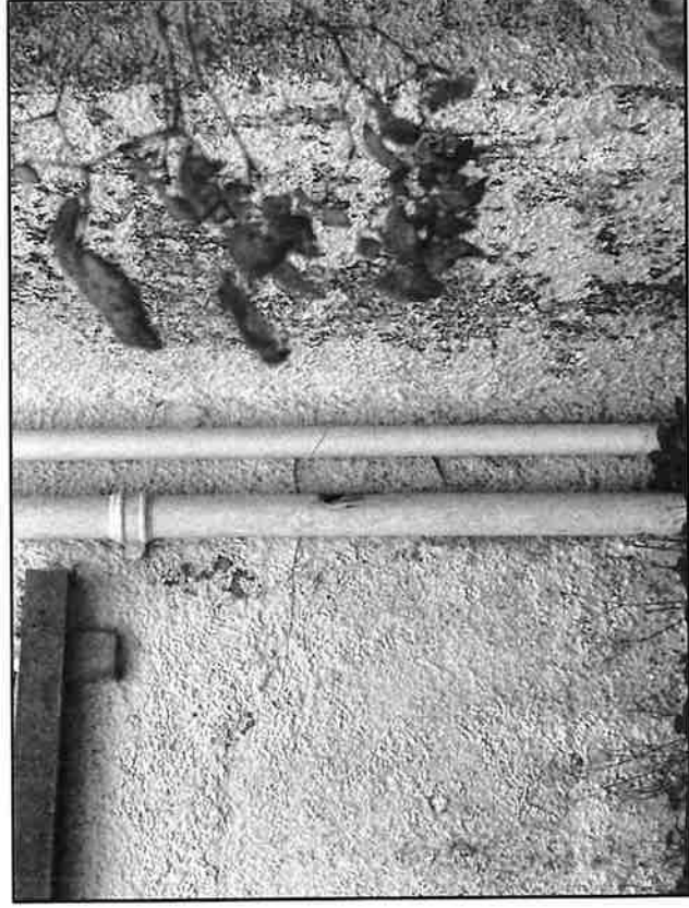
021. Hole due to corrosion to cast iron down pipe at rear elevation adjacent to equipment store
