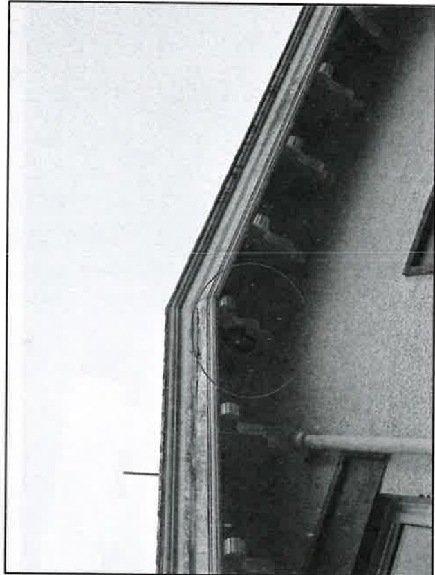
035. Section loss to decorative timber soffit detail at front elevation
