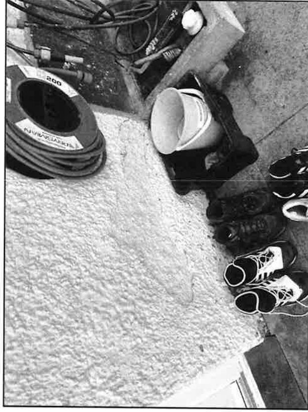
027. Area of spalled render finish at front elevation
