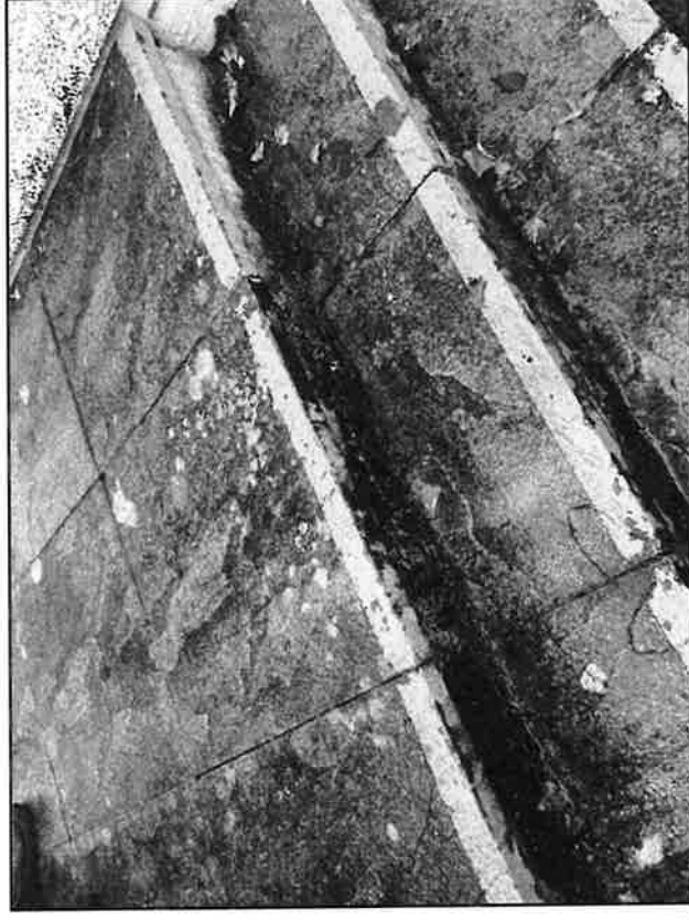
018. Example of paving slabs lifting / loose underfoot
