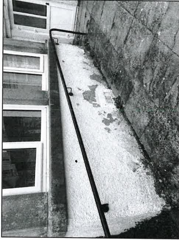
016. Example of flaking paint finish to render at rear elevation
