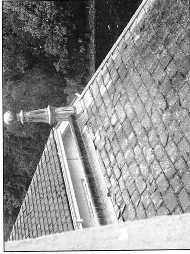
002. Example of damaged slate tiles to roof coverings
