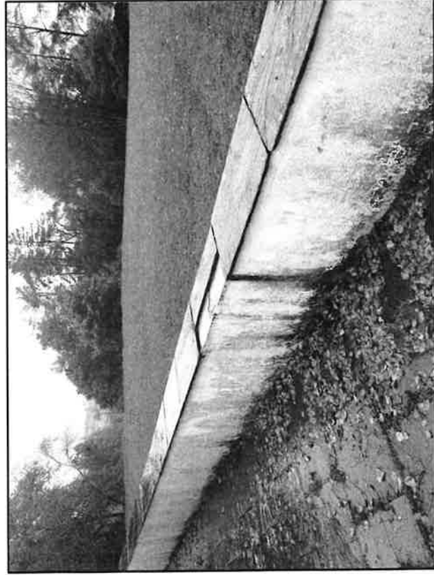
009. Example of missing coping stone to boundary wall
