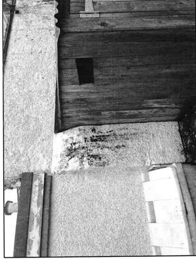
033. Further staining and moss growth to render adjacent to generator at front elevation
