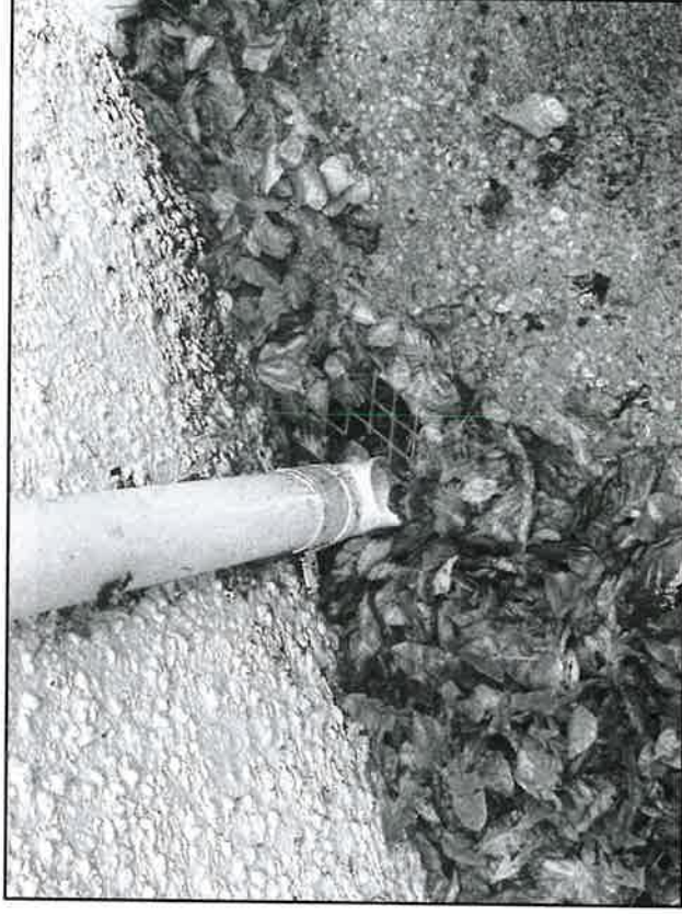
004. Example of gutleys filled with fallen leaves
