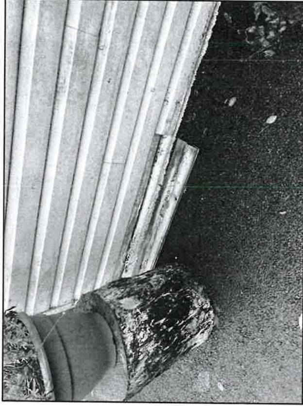
032. Displaced section of timber cladding to front elevation G31 Equipment store
