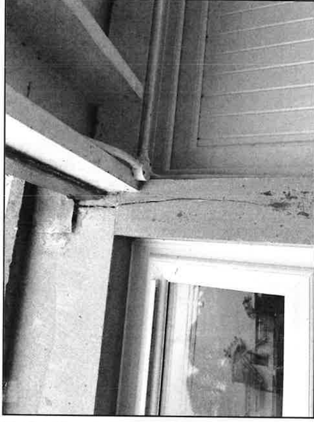
028. Vertical crack, wider at the top, to stone window detail to LHS of front elevation
