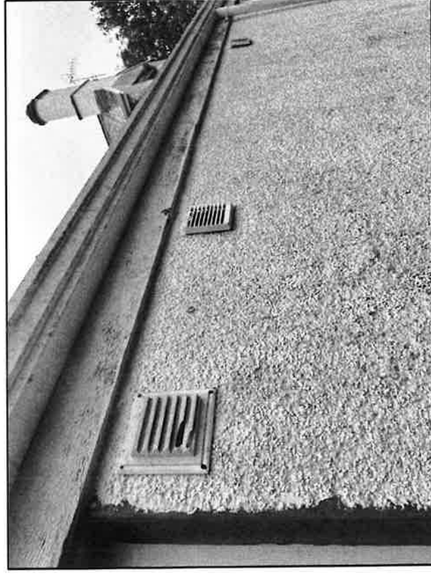
017. Painted timber fascia at rear elevation in poor condition
