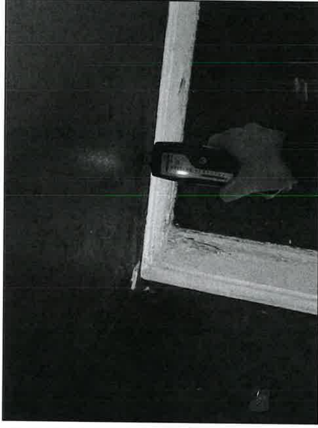
040. High damp readings recorded at front LHS of porch at low level
