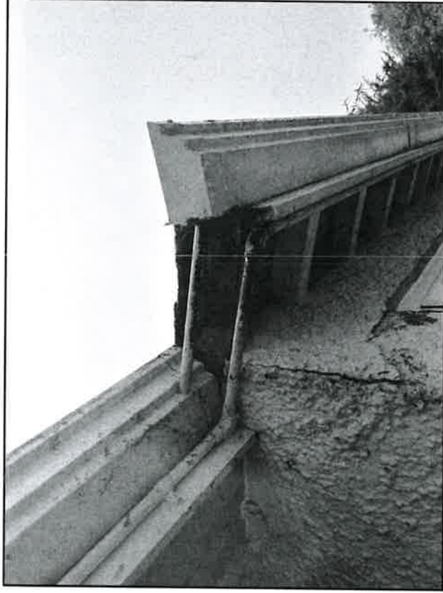
031. Crack to render and missing section of fascia to G29 Laundry Room
