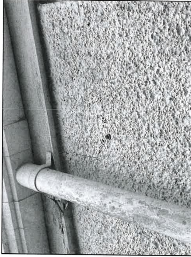
019. Crack to render at rear elevation of one storey bedroom section
