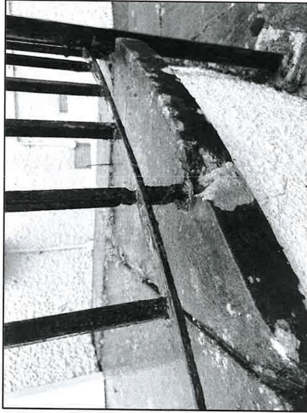
011. Volume loss to few iron fence spindles to dining hall
