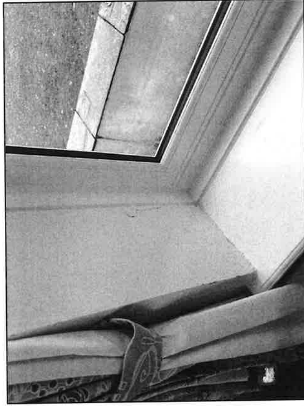
046. Example of non-structural cracking around window reveals, likely to be causing during recent window replacement scheme
