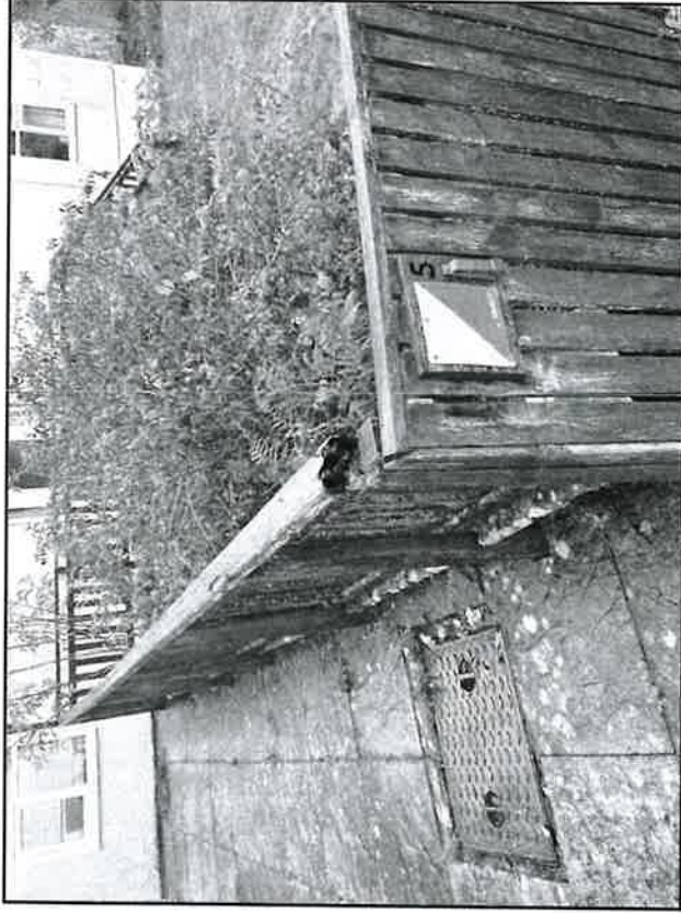
015. Volume loss of timber handrail due to rot at rear elevation
