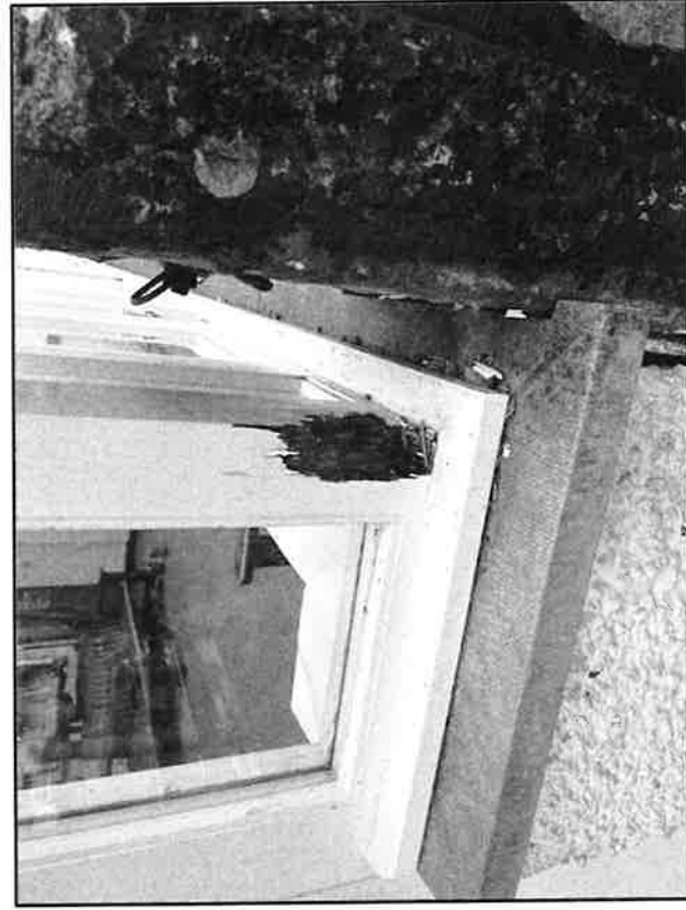
029. Volume loss of timber window unit due to rot to conservatory
