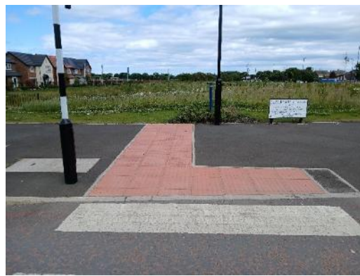
Pedestrian crossing with tactile paving and dropped kerb for inclusive access.
