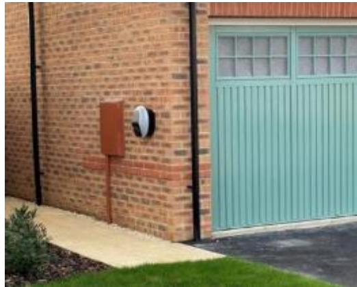
Electric vehicle charge point positioned on the side elevation.
